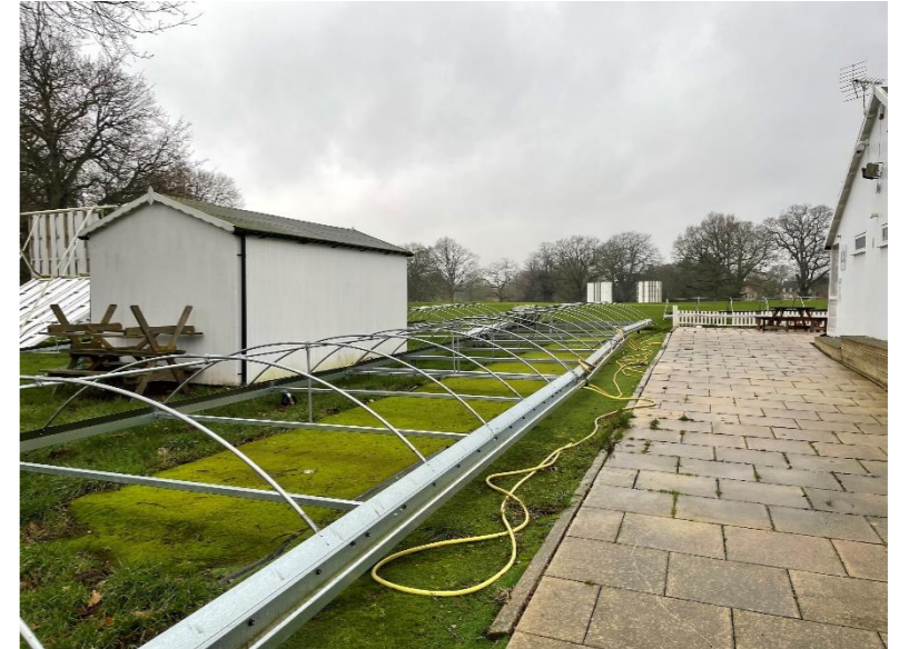
Exposed equipment with no storage facility
